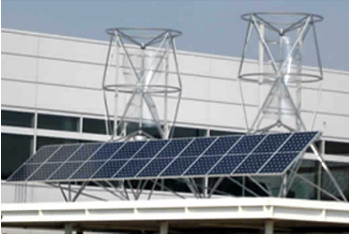
Figure 17. Hybrid wind and photovoltaic solar installation of vertical helical 610V2 turbines.
